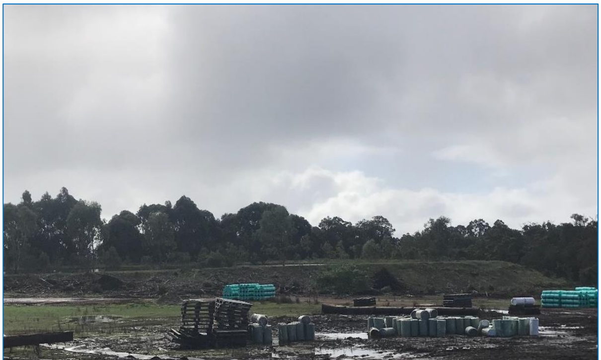
Figure 6 – Evidence of Clearing in Plot 11 (Image Looking North)
