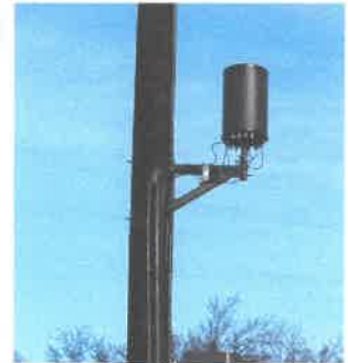
5G 'small cells' are rapidly being installed on streetlights, electricity poles, on trees and park benches; they cover 100-300m ranges; are lower powered, and still hazardous.
