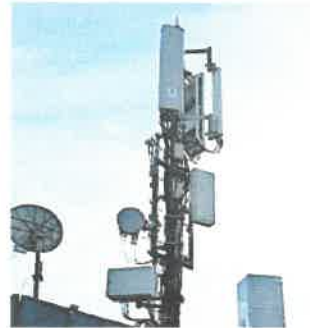
5G masts are being erected on top of residential apartments, office blocks, building facades, every 1-2km apart. These have high transmission powers and kilometer ranges.
