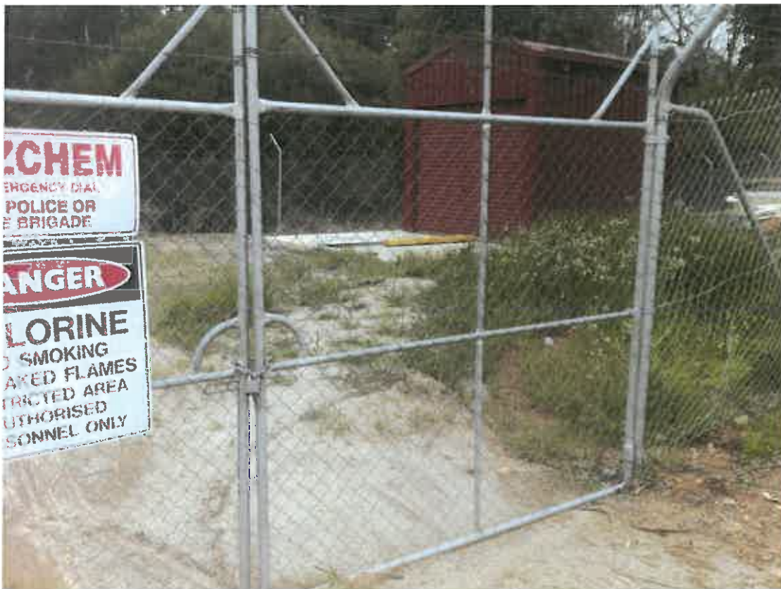
Chlorine gas storage facility
