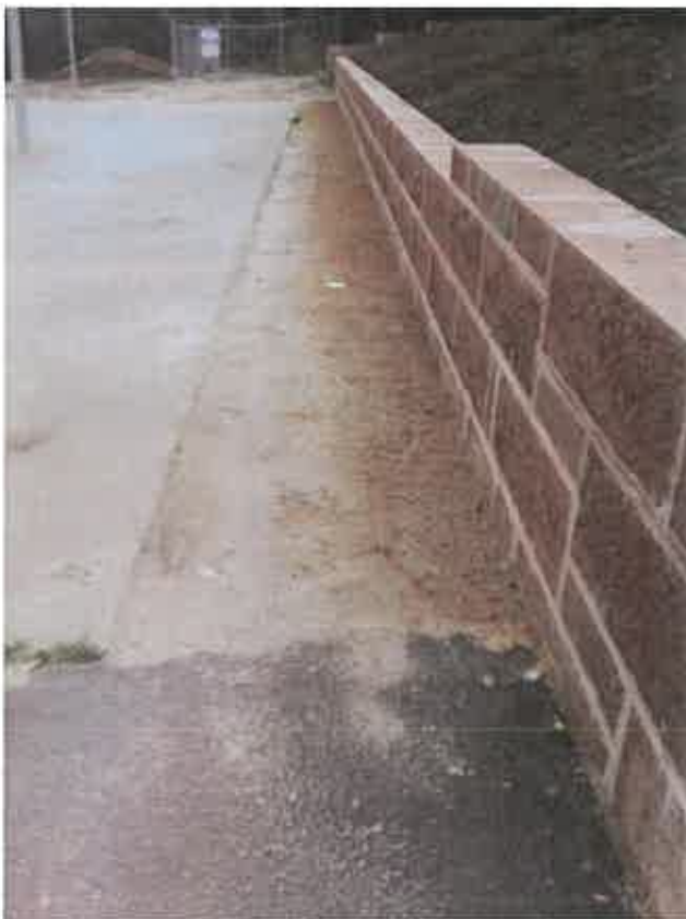
Area at the bottom of the new retaining wall (where the path alongside the toilets finishes) looking north toward the gas chlorine storage facility.
