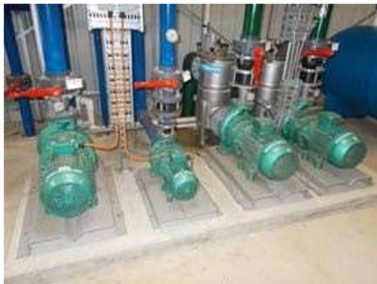
Figure 28 Filtration and feature pump motors
